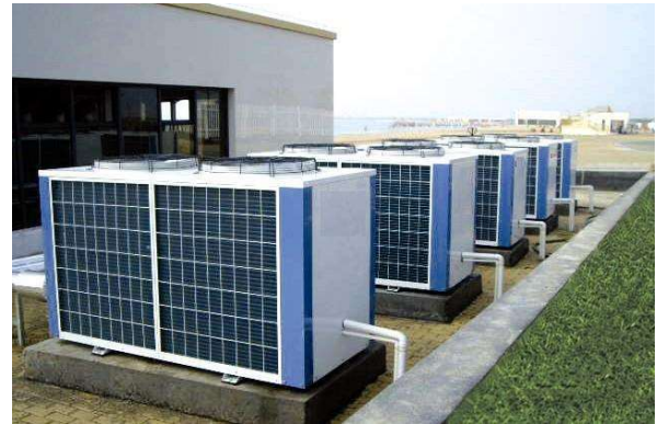
Figure 7: Outdoor units of ASHP – at Ringer’s Road it is expected these will be surrounded by an acoustic enclosure.
