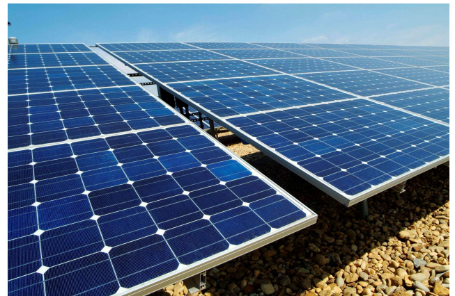
Figure 5: Monocrystalline PV arrays
