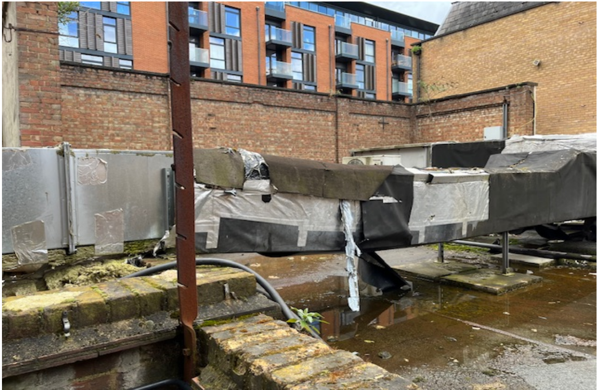
View of roof / parapet wall of 2-4 Ringers Rd with flank elevation of No.6 Ringers Road in view standing in south western corner of SA grounds
