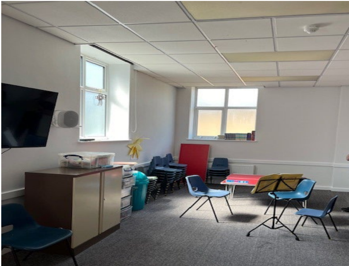
Window in western flank wall at rear of SA (children's room) and rear elevation window
