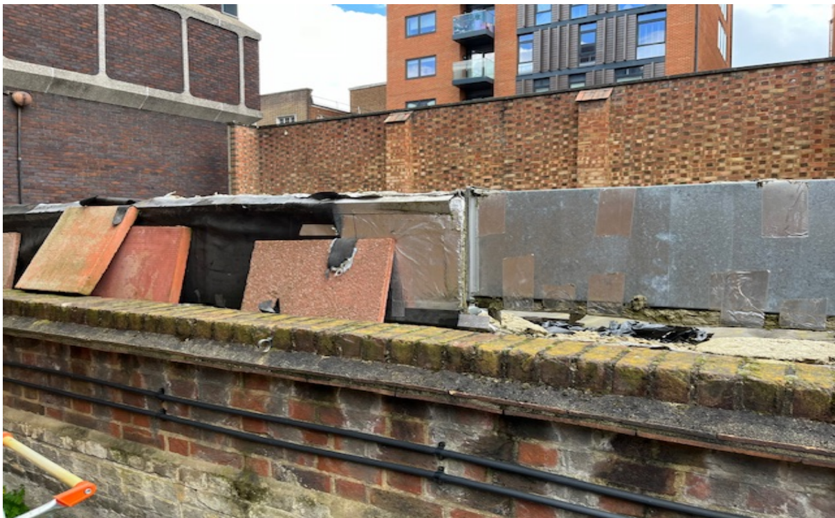
Rear elevation of No.64 H/s, 2-4 Ringers Road parapet wall, Henry House in background
