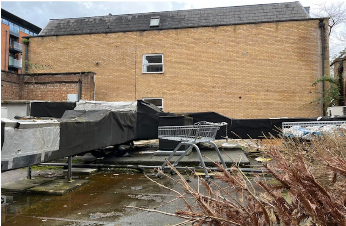
View looking across roof of 2-4 Ringers Rd toward flank elevation of No.6 Ringers Road
